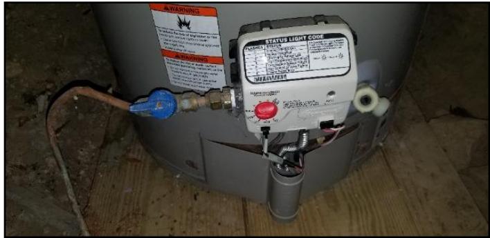
No drip leg (sediment trap, dirt pocket)
