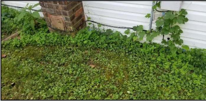
Improper slope or drainage
