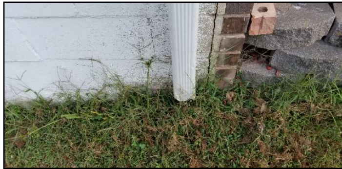
Should discharge 6 feet from building
