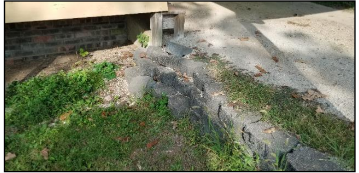
Improper slope or drainage
