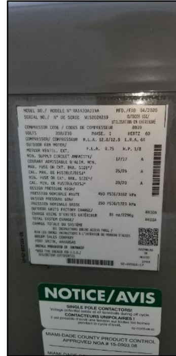
No air conditioning or heat pump...
