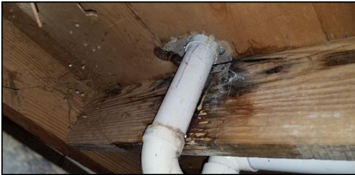
Affected by Moisture.
