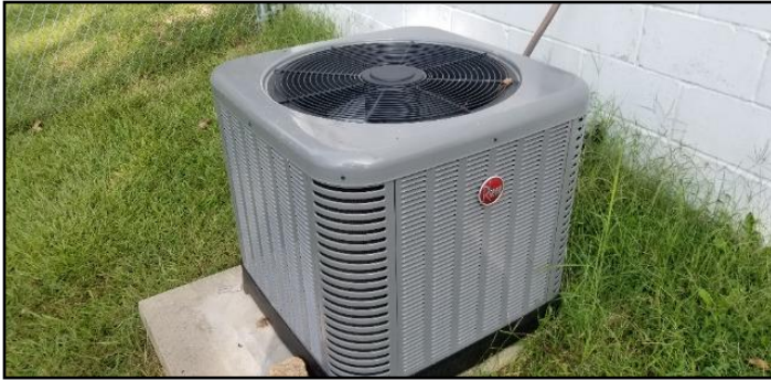
No air conditioning or heat pump...
