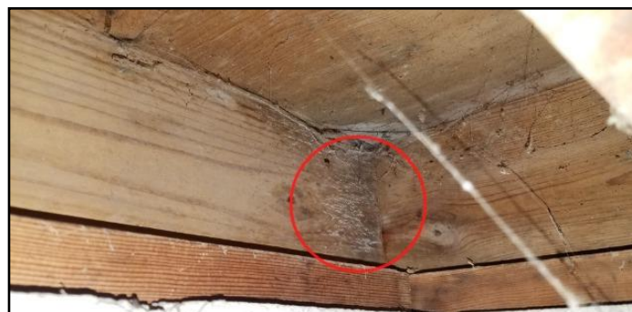
Affected by Moisture.
