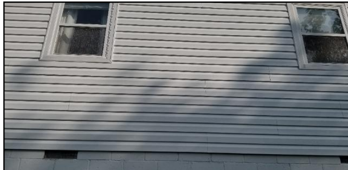
Paint and Caulking - deteriorated / missing
