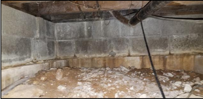
Moisture against that uphill wall.
