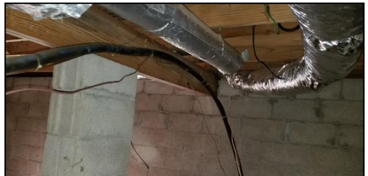
No air conditioning or heat pump...
