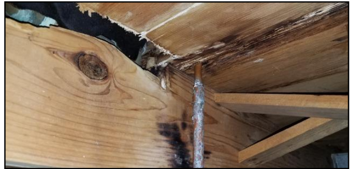
Affected by Moisture.
