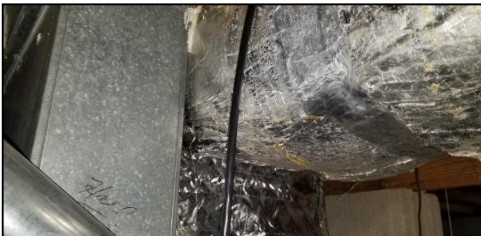
No air conditioning or heat pump...
